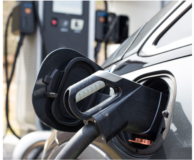
Electric vehicle charging station, South Korea
